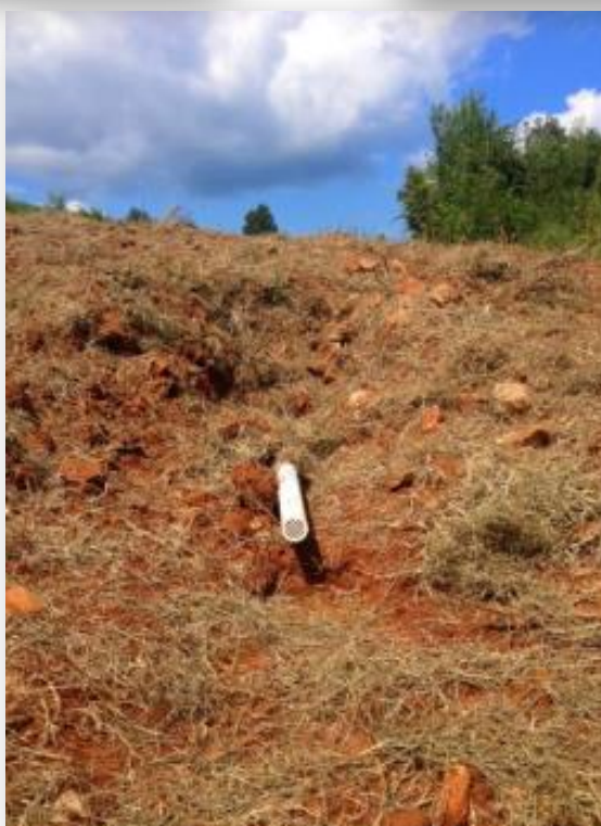
Figure 2. Trench construction and interceptor pipe installation adjacent to the manure holding ponds at the C&H Farm, Mt. Judea, Newton County.
